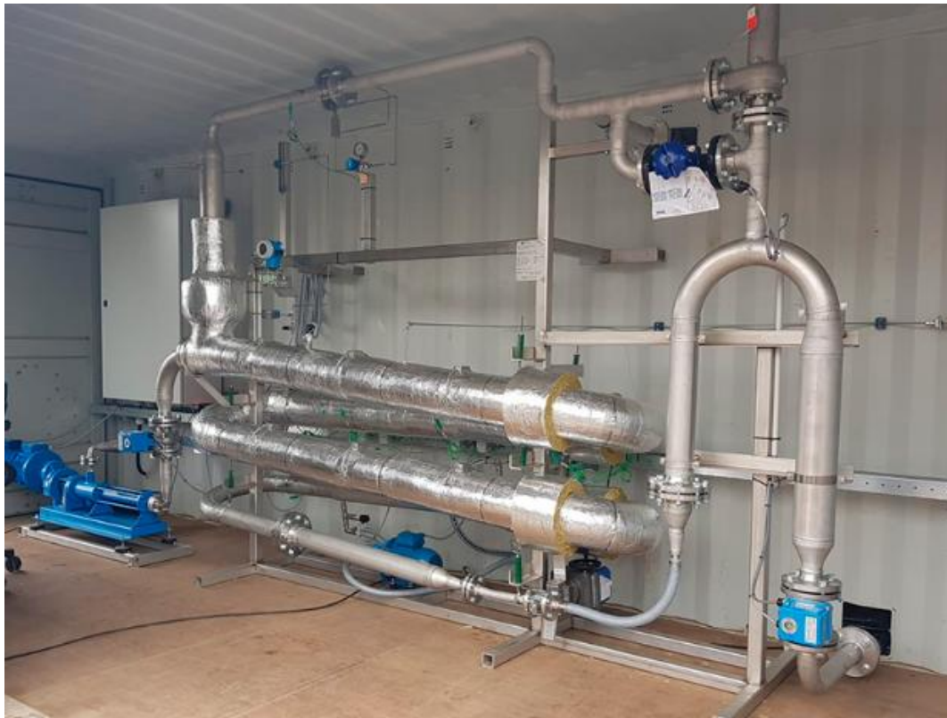
TORWASH® hydrothermal treatment of paper sludge
